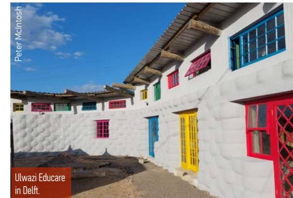
Building walls using tyres with ecobricks to fill spaces at Ulwazi Educare.
