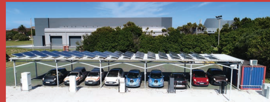
The uYilo smart grid ecosystem facility in Port Elizabeth is already demonstrating local activities of smart grids with EVs – solar charging optimisation, second life EV batteries, vehicle-to-grid, and autonomous energy management.
